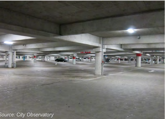
Garages lacking wayfinding can be confusing for users and may deter people from utilizing available garages.
